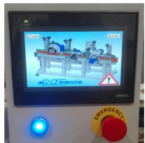
PANEL DE CONTROL/ CONTROL MACHINE
